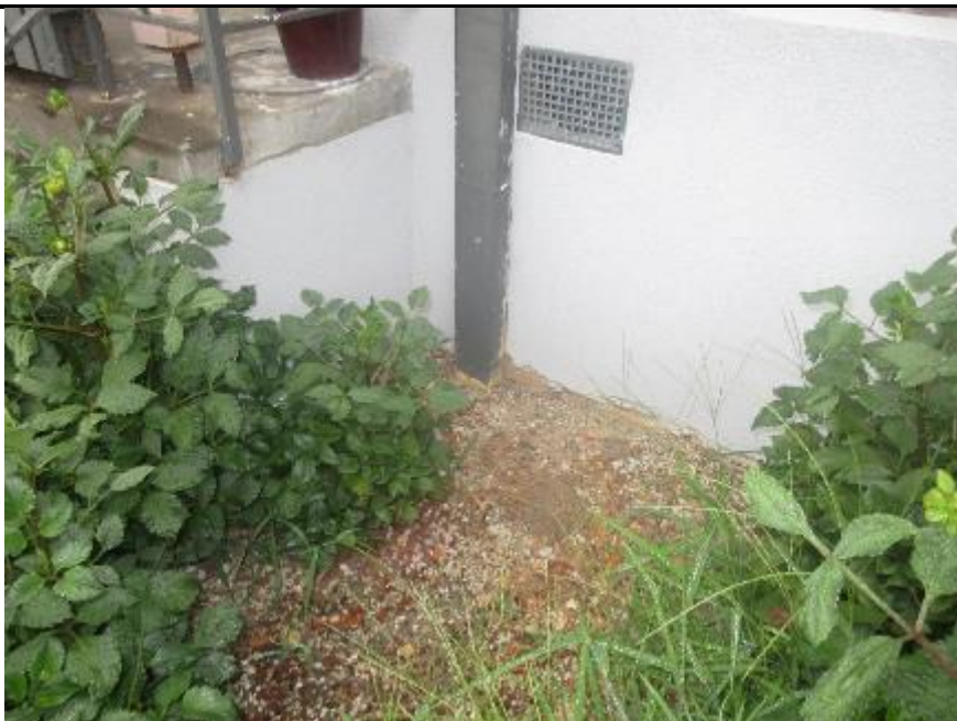
Photograph 18. Downpipe along west side elevation upstream of broken stormwater drain.
