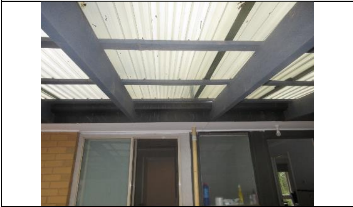
Photograph C3. Sagging to timber purlins.
