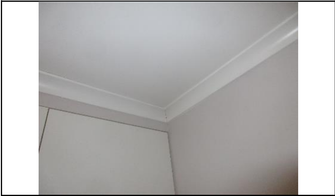
Photograph 3. Typical hairline crack to mitre joint of ceiling cornice.
