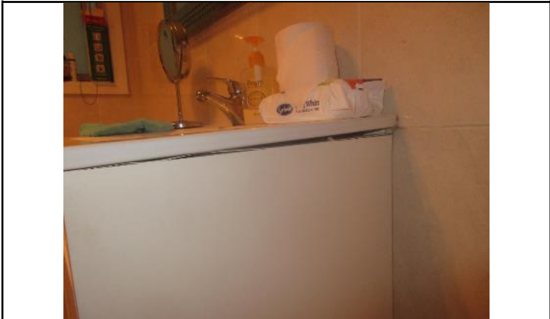
Photograph 5. Separation along vanity unit side / bench top junction.
