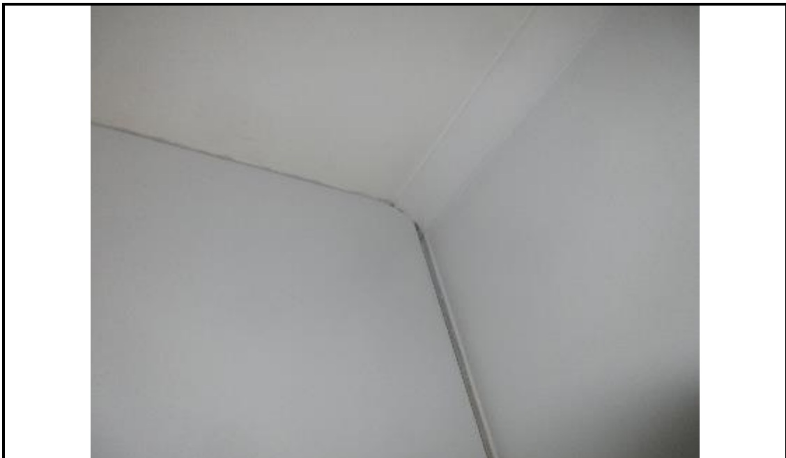
Photograph 8. Separation of bedroom 1 built in robes from the wall.
