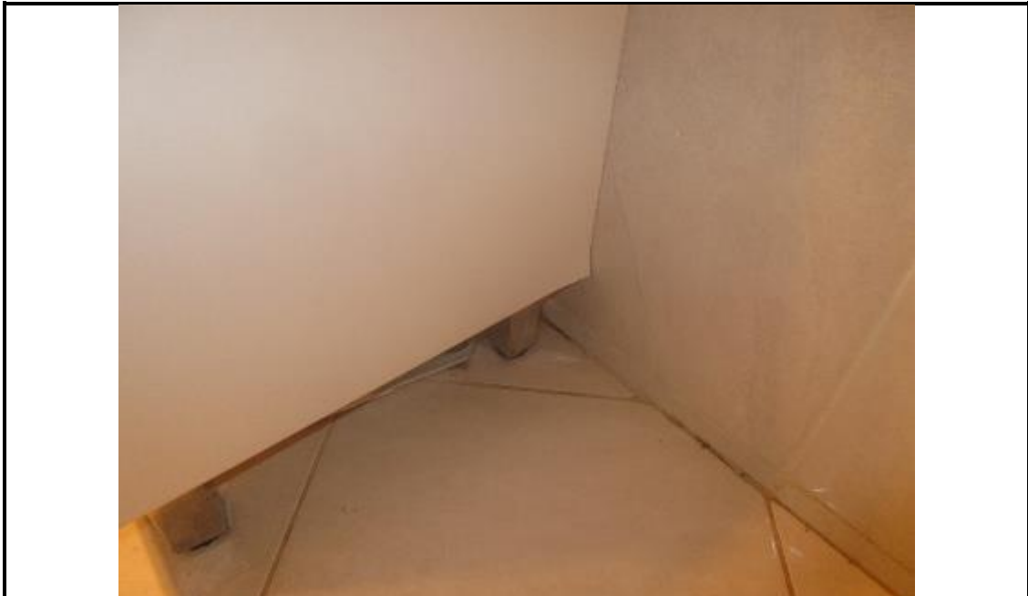
Photograph 7. No movement at floor / wall junction below vanity unit.
