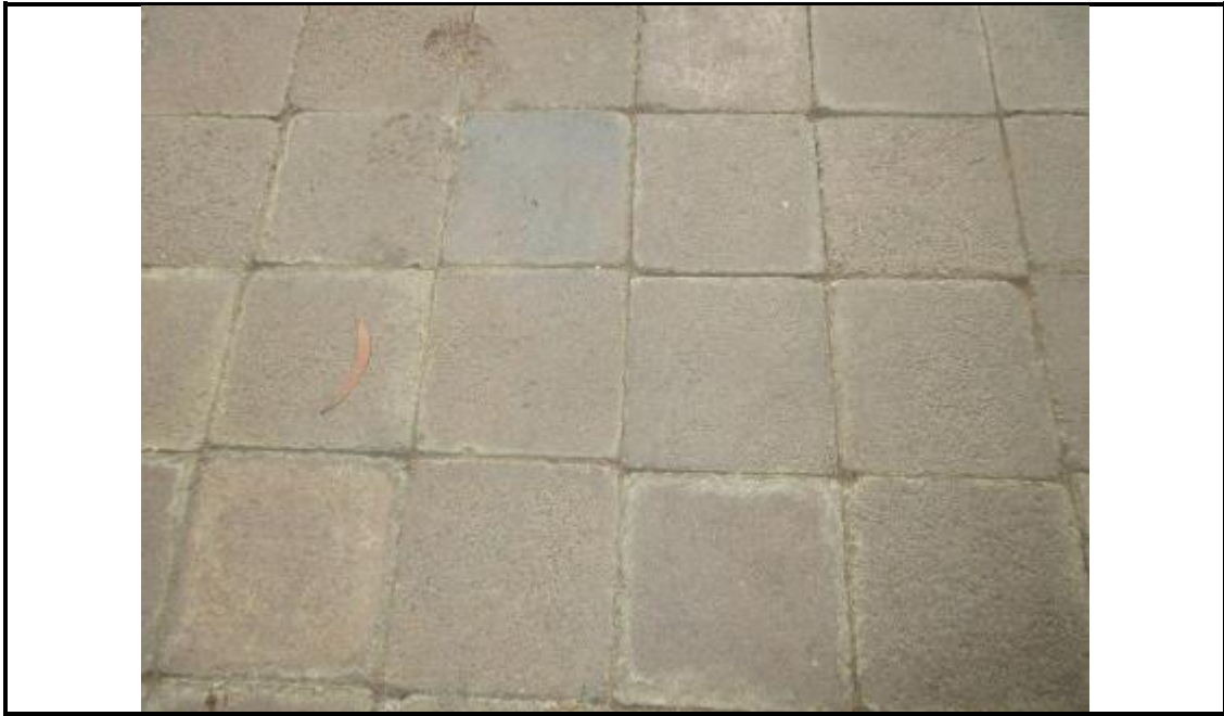
Photograph B7. Bedding joints misaligned.
