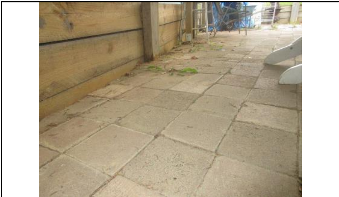
Photograph B6. Undulating level across the surface of the paved area.
