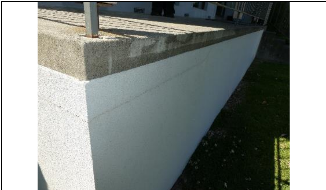
Photograph 14. Crack below porch slab (site visit 15 April 2020).
