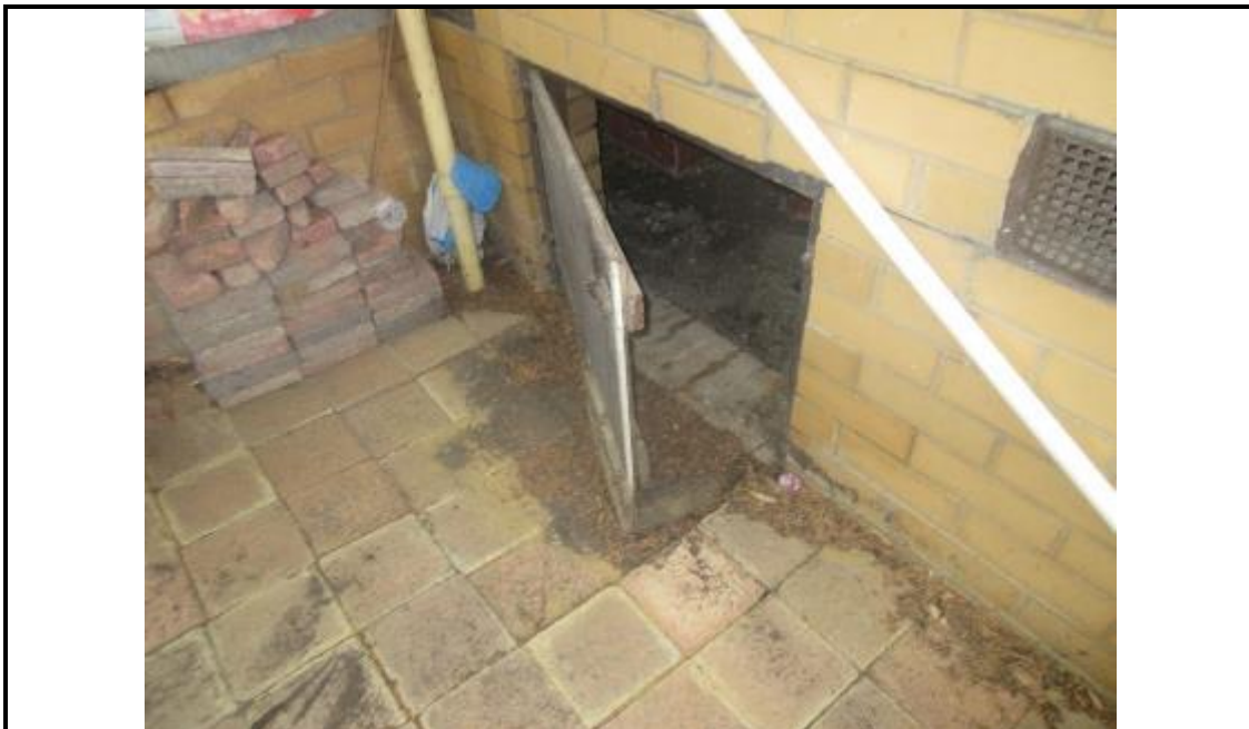
Photograph B4. Sub-floor access door no longer opens fully.
