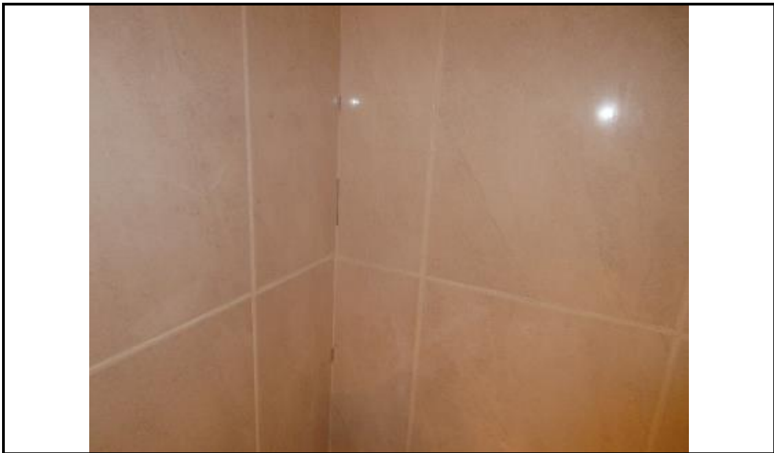
Photograph 4. Damage to tile grout in bathroom.
