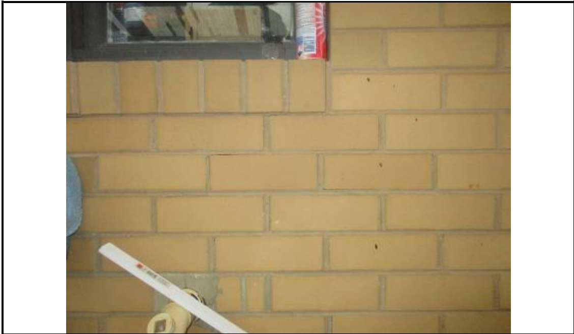
Photograph 11. Crack along east side elevation.
