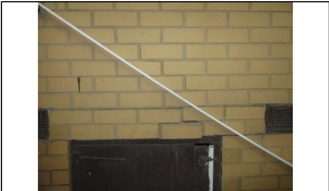
Photograph 10. Crack above sub-floor access door, note no steel lintel above door to support brickwork.
