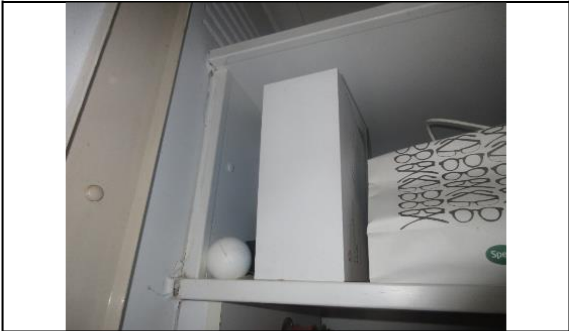
Photograph 9. Separation of bedroom 1 built in robes from the wall.
