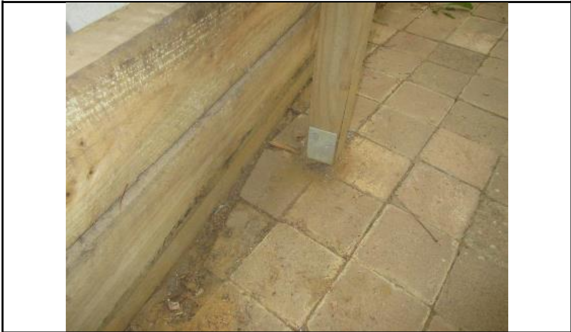
Photograph B5. Mismatched edging to unit pavers.
