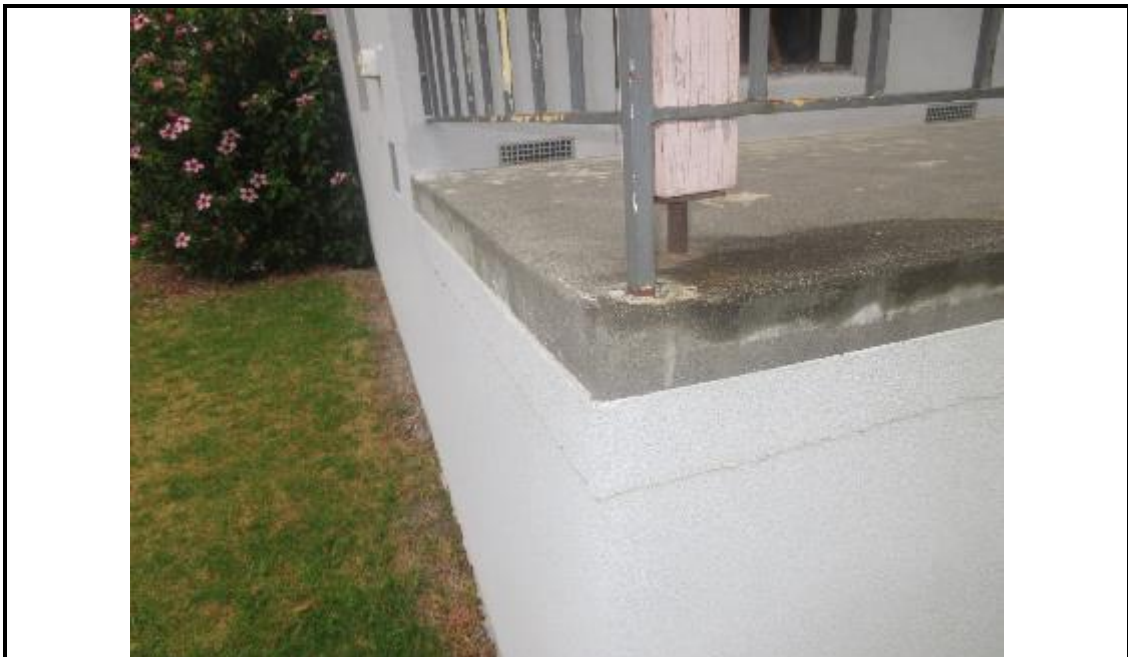
Photograph 12. Crack below porch slab.
