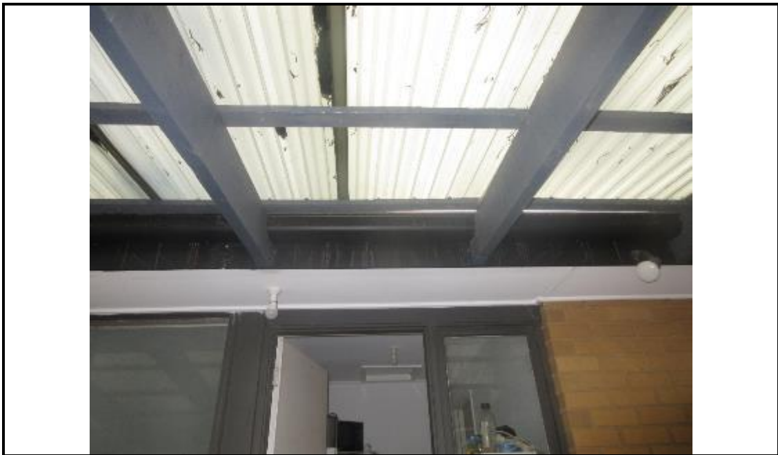
Photograph C4. Sagging to timber purlins.
