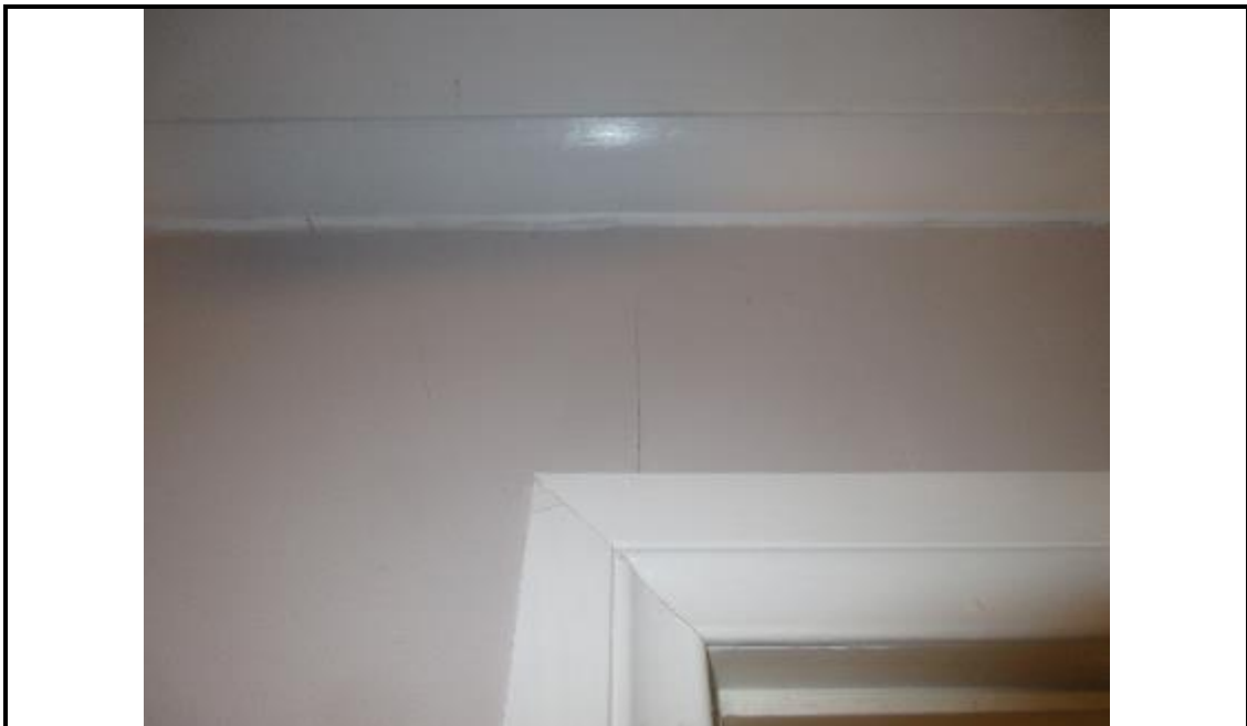
Photograph 2. Typical hairline crack to wall lining (in rear south-east bedroom).
