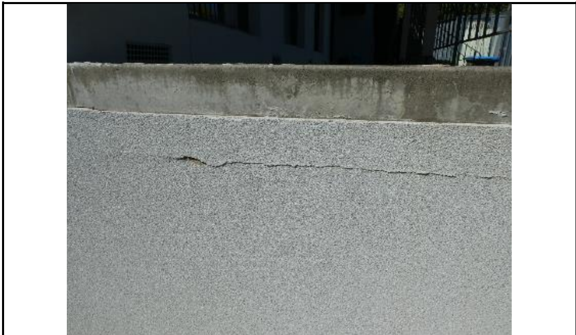
Photograph 15. Crack below porch slab (site visit 15 April 2020).
