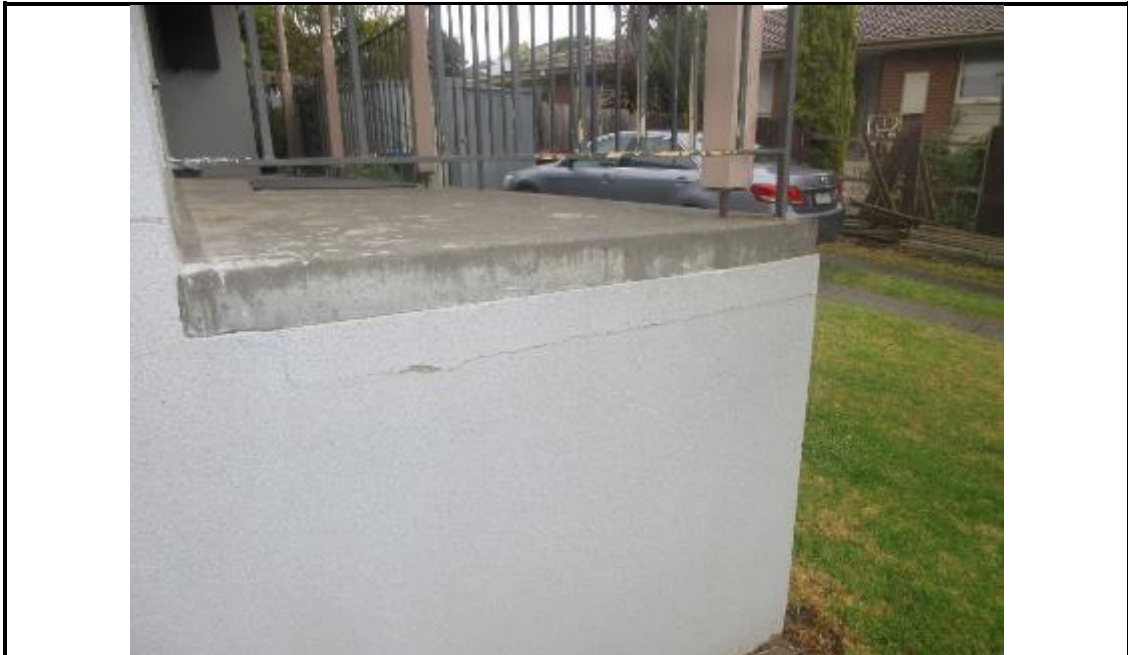
Photograph 13. Crack below porch slab.
