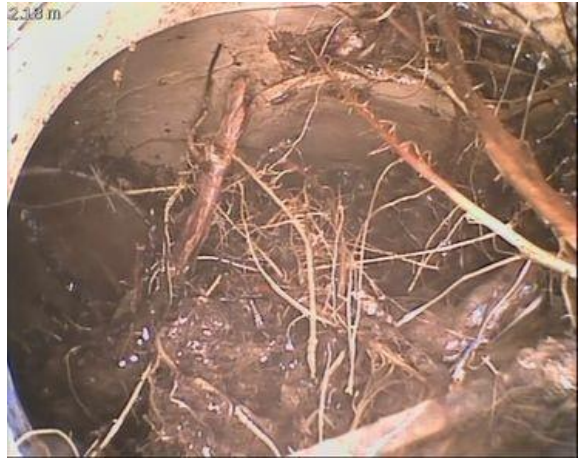
TREE ROOT IN DRAIN
