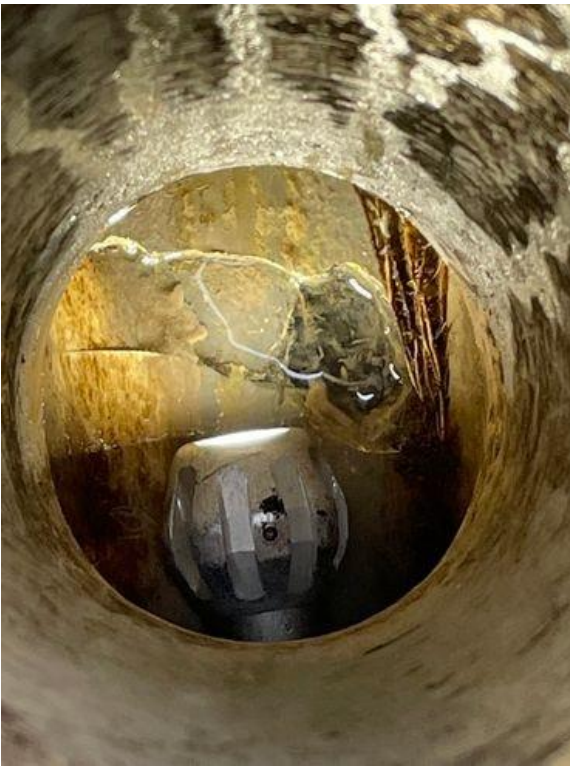
TREE ROOT IN DRAIN
