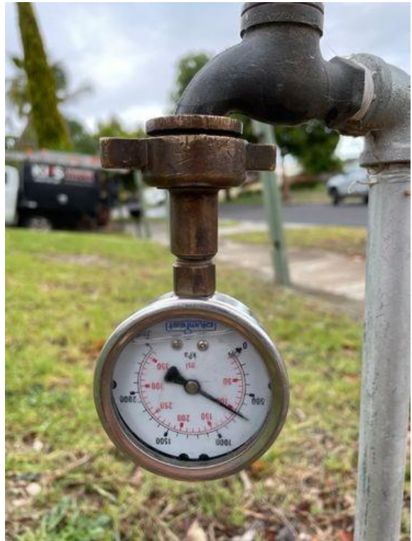
MAIN LINE WATER PRESSURE
